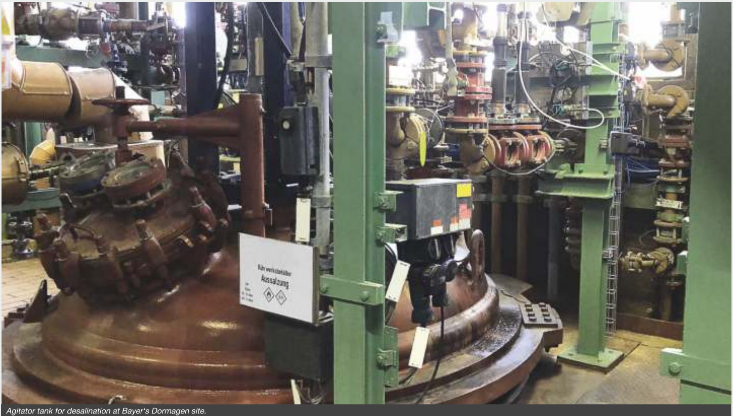
Agitator tank for desalination at Bayer's Dormagen site.
