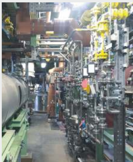
Process technology plants, such as those at Bayer in Dormagen, are generally highly sophisticated and designed for a very long service life.
